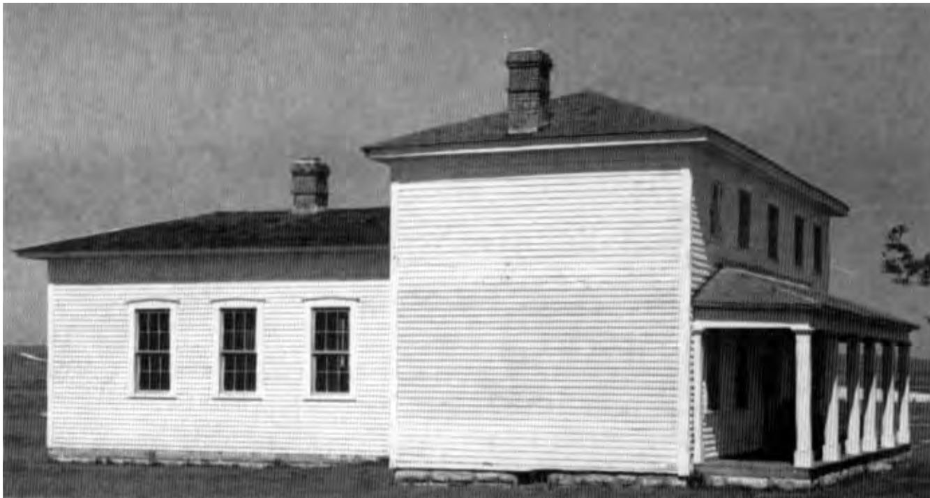
In a project at Fort Hays, Kansas, the wood frame officers' quarters were restored to the late 1860s—their period of significance. This included replacing a missing kitchen ell, chimneys, porch columns, and cornice, and closing a later window opening in the main block. The building and others in the museum complex is used to interpret frontier history.
