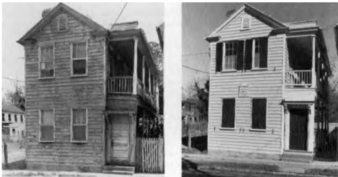
Maximizing retention of historic materials and features is the primary goal of Preservation as demonstrated here in these “before” and “after” photographs. Aside from some minor repairs and limited replacement of deteriorated material, work on this house consisted primarily of repainting the wood exterior. Photos: Historic Charleston Foundation.
